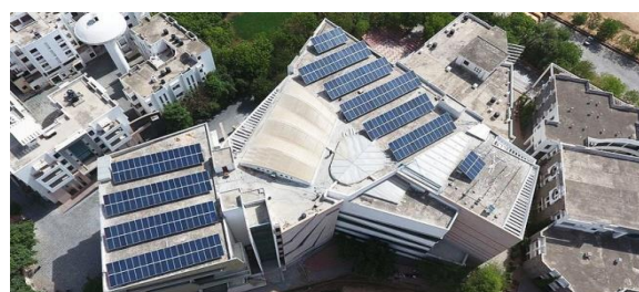
Fig. 4 120KW Solar Power Plant in SGVU, Jaipur
