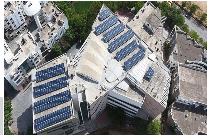
Fig. 6 120KW Solar Power Plant in SGVU, Jaipur
