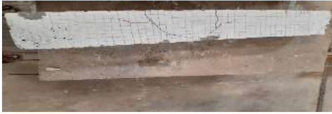
Figure 5. crack pattern of GPC beam
