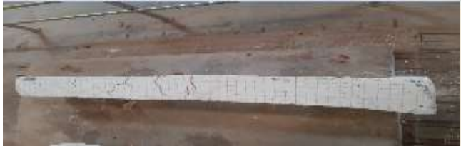
Figure 6. crack pattern of rcc beam
