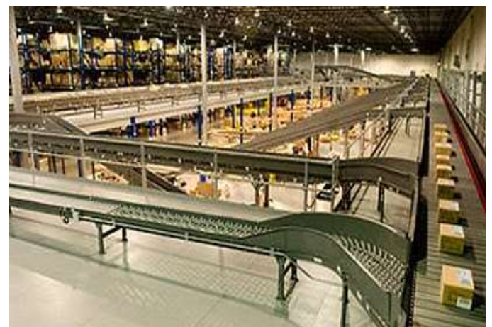
Fig.1.11 Integrated Material Handling System
