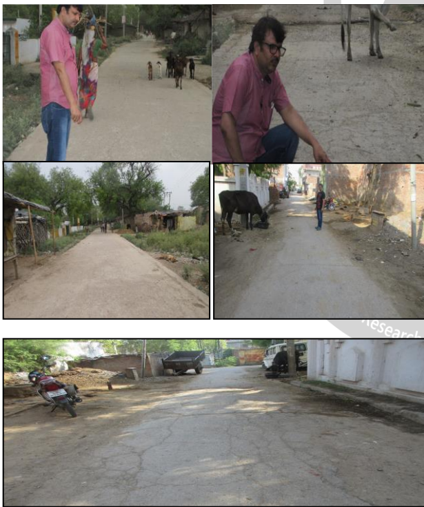
Fig: 1 Photographs of different c.c. roads which shows crocodile crack
