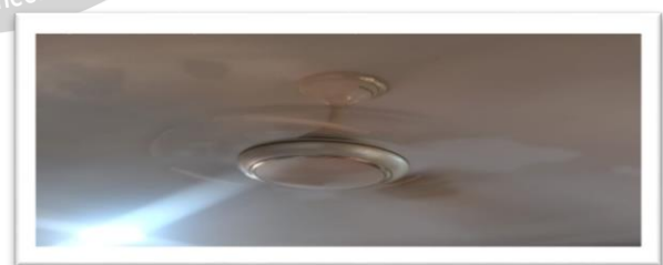
Fig. 9 Fan on (after knock)
