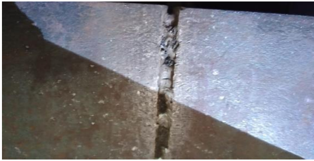
Incomplete fusion metals.
