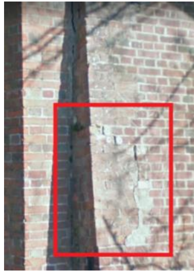
Fig. 6. Stepped Cracking & ongoing Maintenance
