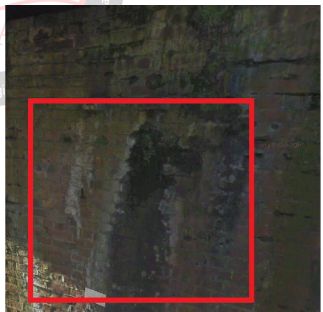
Fig. 8. Water Strains / Wet patches
