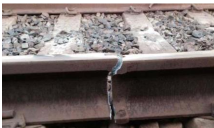
Figure 1: Cracks in Railway Track.
